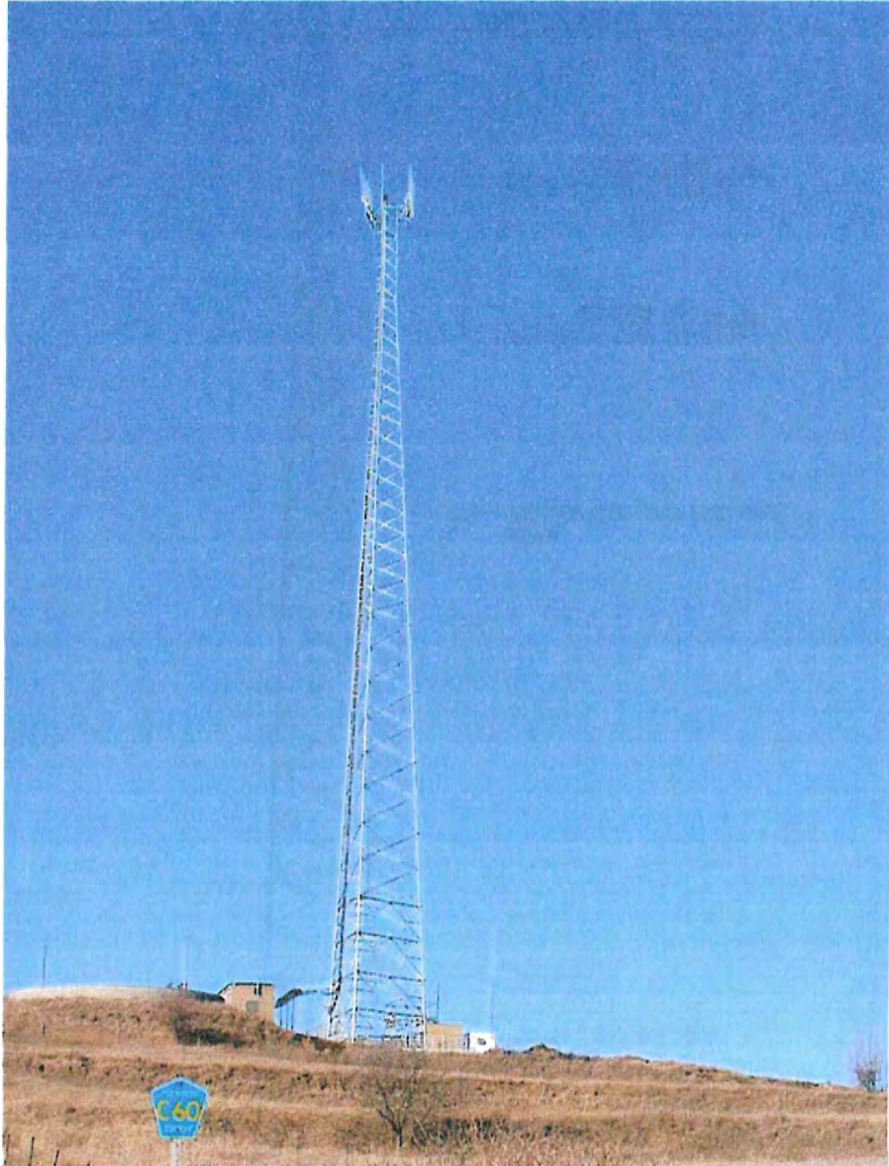
250' tall tower with ground equipment, driveway and fencing
