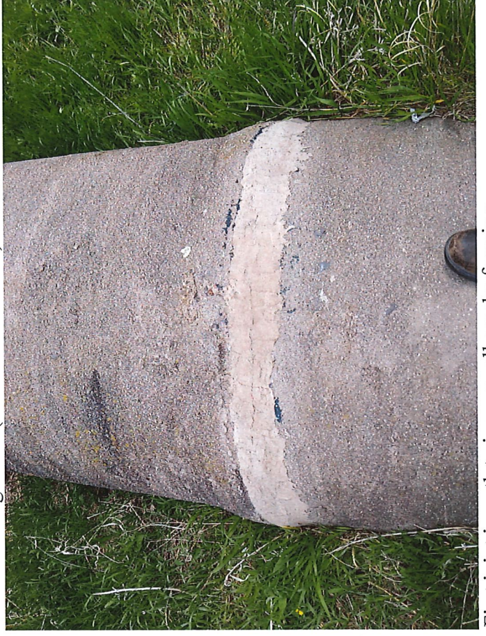
First joint in outlet pipe – small cracks forming
