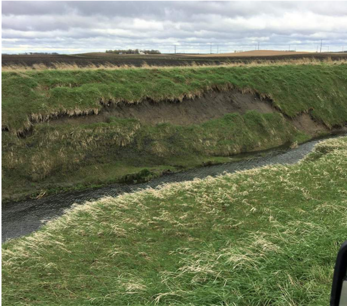
Example of damaged ditch site needing repair
