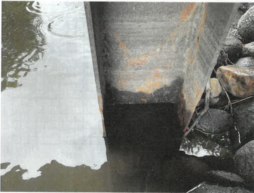
Section loss noted on south pier piling on bridge 64503.
