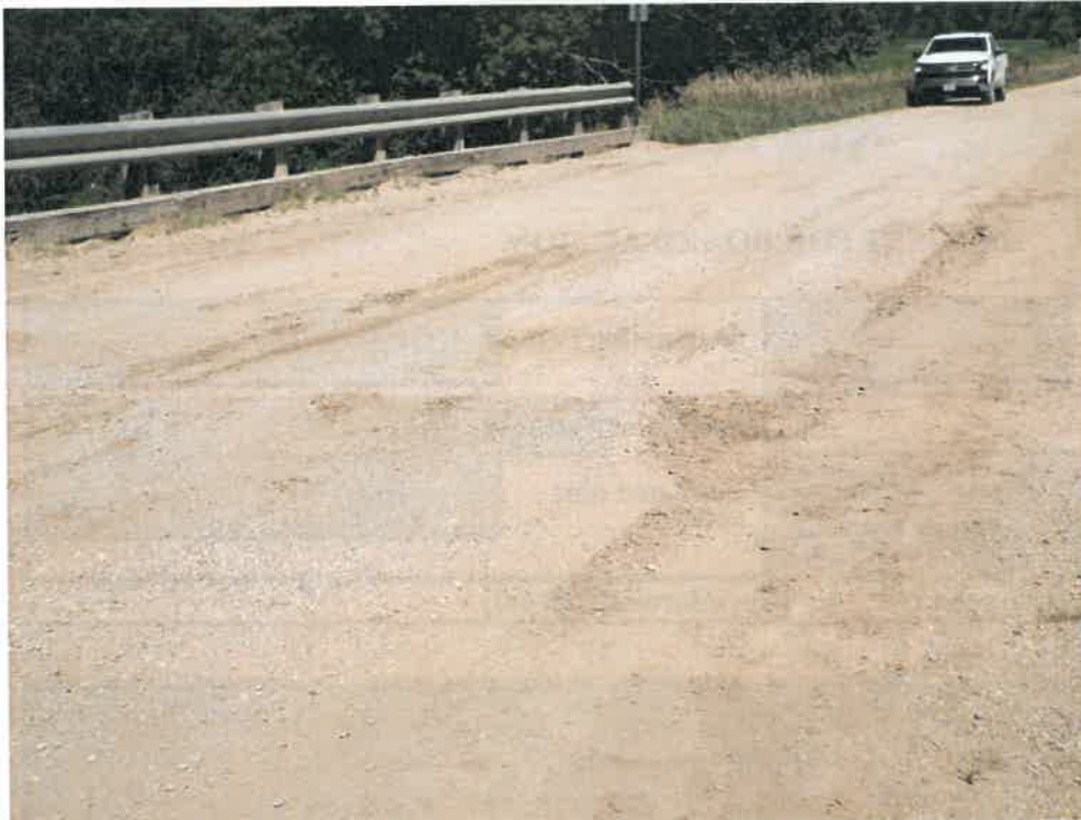
Initial deflection noted by maintenance forces over bridge 64503. Facing northwest.
