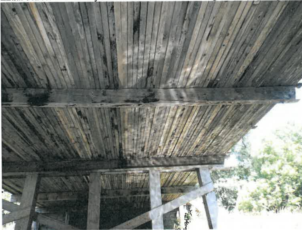
Fractured timber floor beam on br 64503. Facing north.
