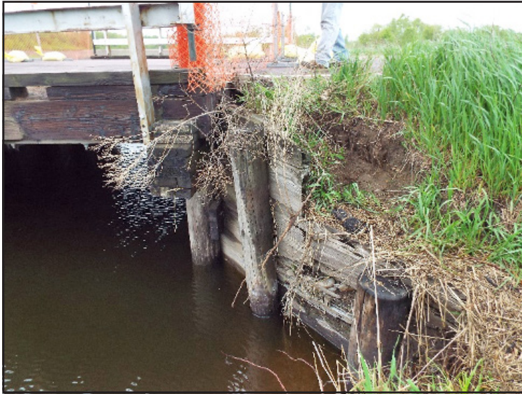
CSAH 8 Bridge 89825 replacement that occurred in September 2022. Note the advanced deterioration of the abutment and abutment pile caps.
