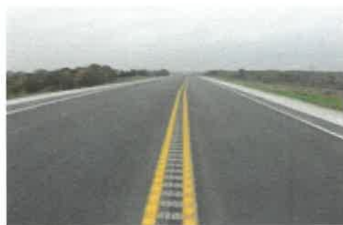
Centerline Rumble Strips
