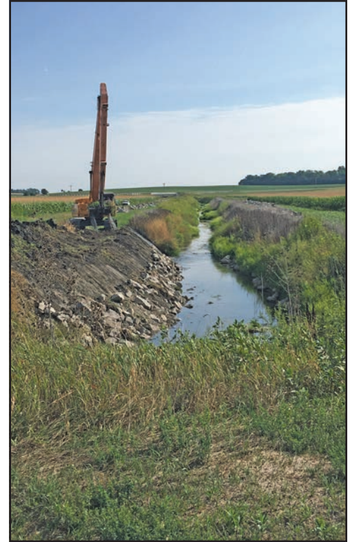
Repair work has begun, but sloughing ditch banks can be seen past the excavator.
