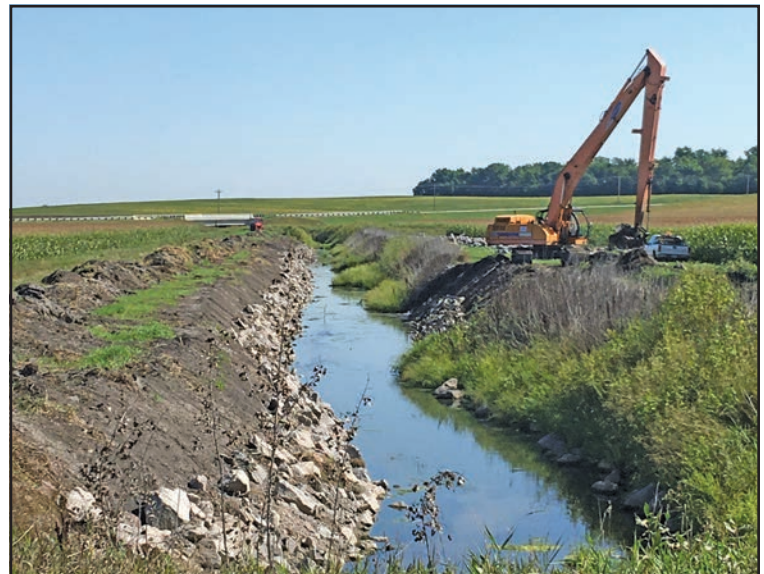
Repair work completed on the left side of the ditch bank. Material has been removed from the ditch and the banks have been hard armored.
