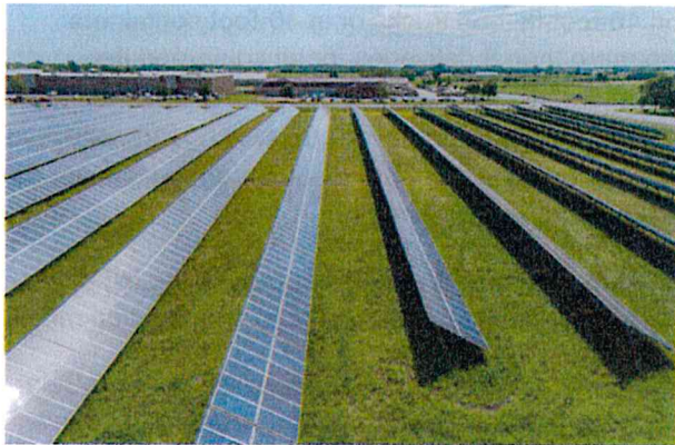
EXAMPLE OF A SOLAR PROJECT IN OPERATION
