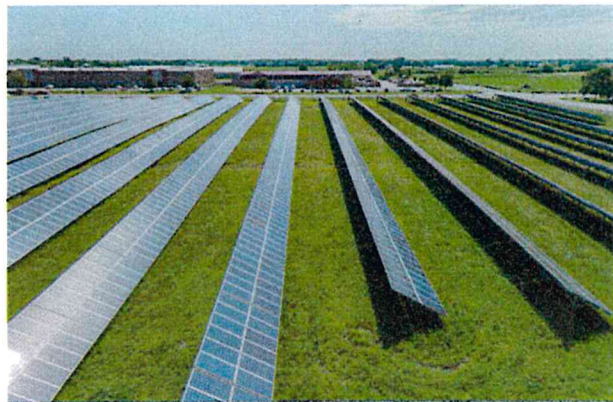
EXAMPLE OF A SOLAR PROJECT IN OPERATION
