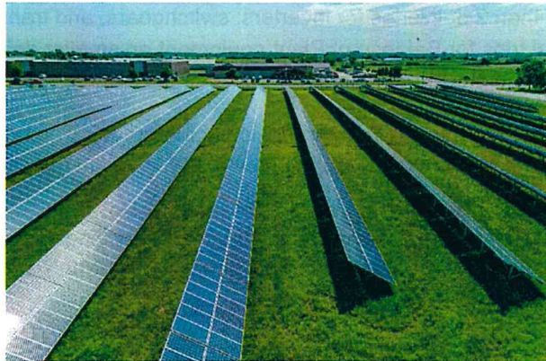
EXAMPLE OF A SOLAR PROJECT IN OPERATION
