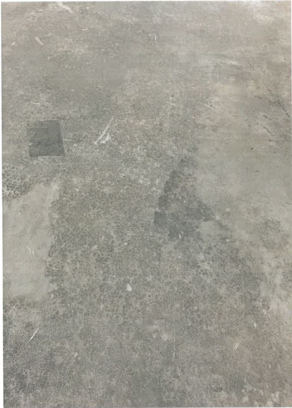
12/16/2022 1820 East Bridge Highway Shop Floor Condition (un-treated areas)
