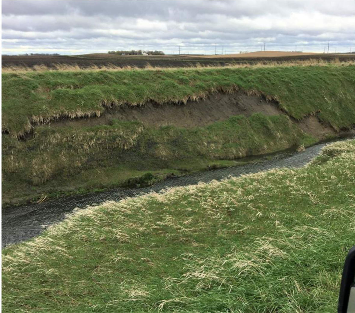
Example of damaged ditch site needing repair
