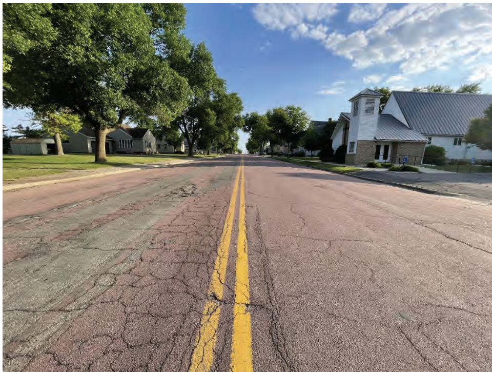
CSAH 7, North of Marion Street, Facing North. Note rutting in tire paths, longitudinal cracking and multiple cracking and alligator cracking.
