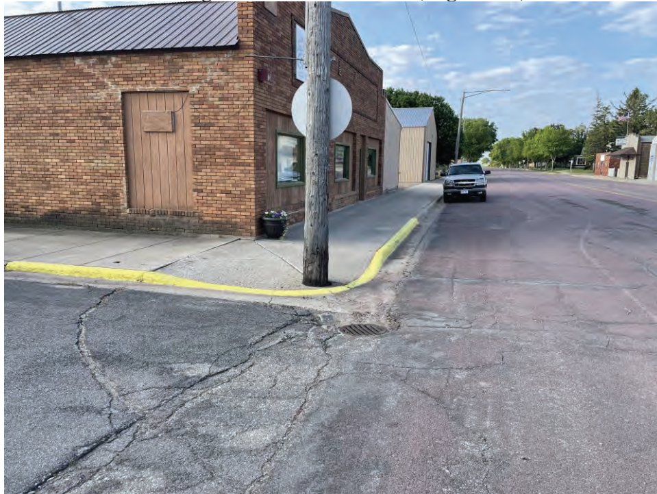
Intersection Quadrant of CSAH 7 and Hibbard Avenue, facing south-southeast. Note non-compliant pedestrian ramp (typical).
