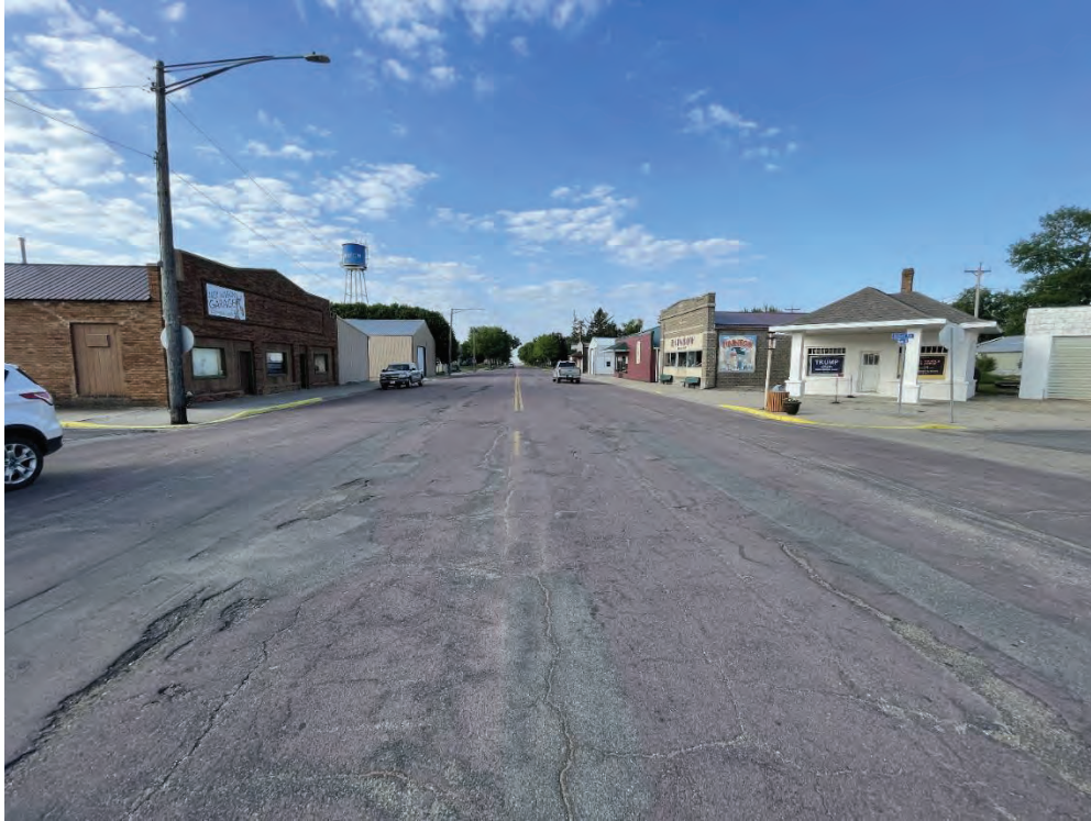
Intersection of CSAH 7 and West Hibbard Avenue – Facing South. Note multiple patches, rutting in tire paths, longitudinal cracking and multiple cracking.
