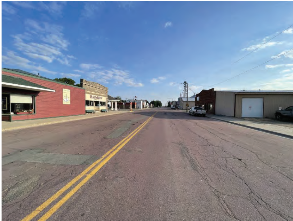
CSAH 7, midblock between West Second and Hibbard Avenue, Facing North. Note multiple patches, rutting in tire paths, longitudinal cracking, multiple cracking and alligator cracking.
