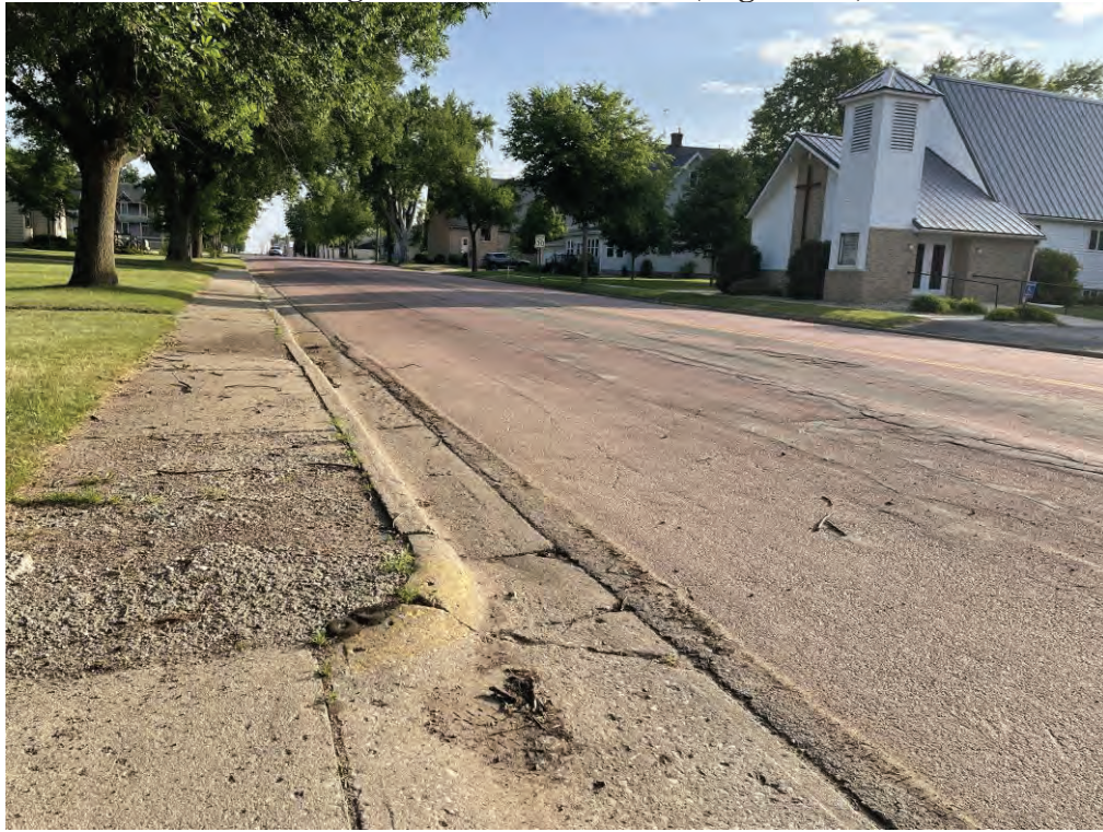
CSAH 7, North of Marion Street, Facing North. Note non-compliant pedestrian ramp and degraded sidewalk condition (typical at various locations).
