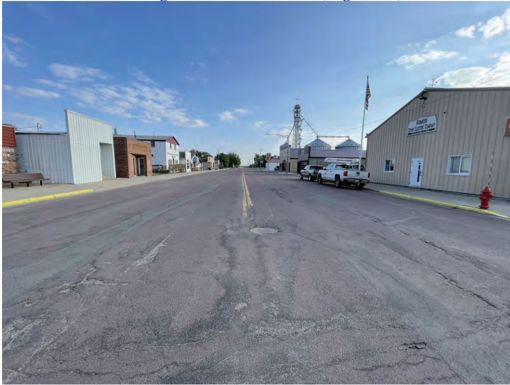
Intersection of CSAH 7 and West Hibbard Avenue – Facing North. Note multiple patches, rutting in tire paths and longitudinal cracking.
