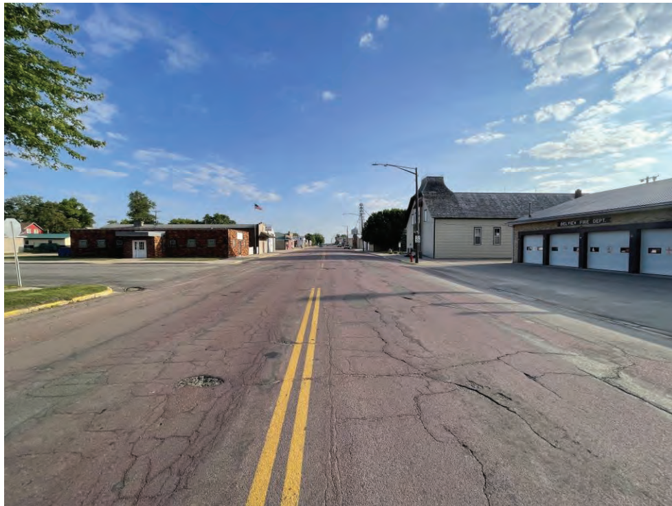
Intersection of CSAH 7 and West 2 nd Avenue – Facing North. Note multiple patches, rutting in tire paths, longitudinal cracking, multiple cracking and alligator cracking.
